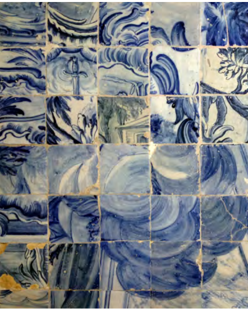
4. This patched section of wall tiles is typical of those seen in churches in Salvador and Cachoiera.
